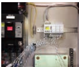
Electricity monitoring device
