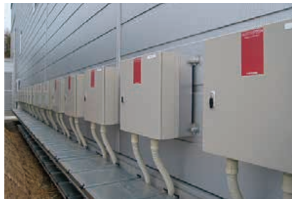
PV Inverters at Fujiyama Works
