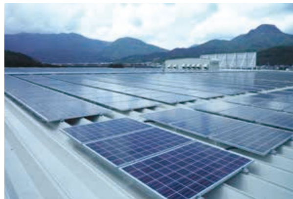
Solar panels at Logistics Center
